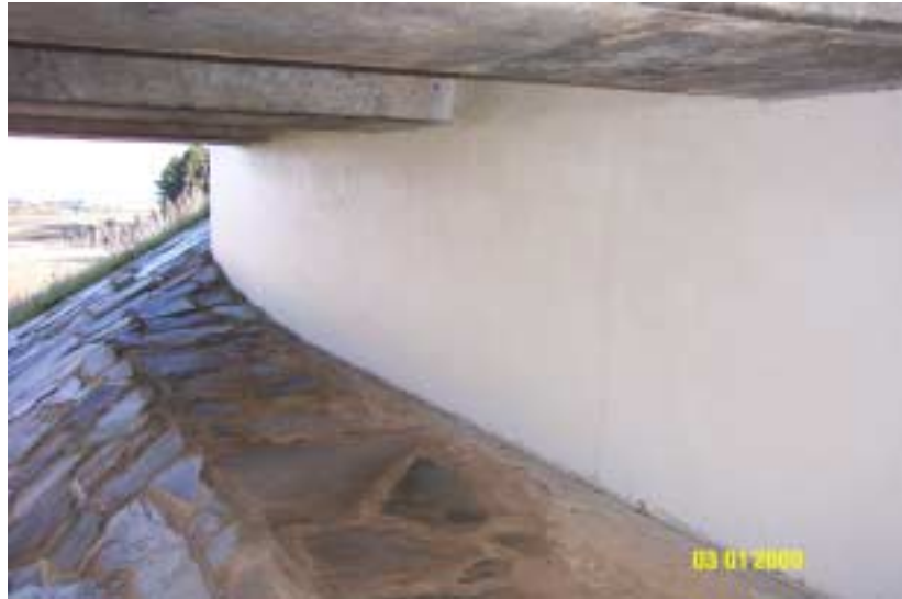
Figure 12: Front of Abutment Showing Condition of Rock Beaching
