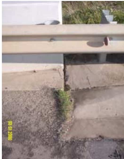
Figure 13: View Showing Gap of Less Than 10mm at End of Abutment
