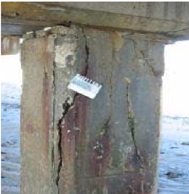
Figure 3: Cracking and delamination in pile induced by corrosion
