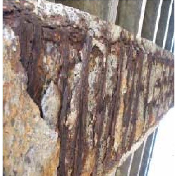
Figure 6: Complete delamination of cover concrete at crosshead soffit
