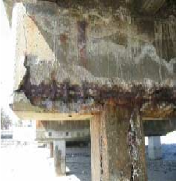
Figure 5: Spalling of cover concrete at crosshead soffit
