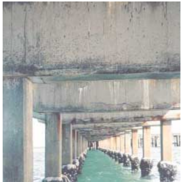
Figure 4: Cracking with rust stains appearing at lower part of crossheads
