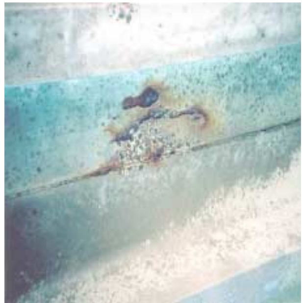
Figure 8: Localised corrosion at the edge of deck plank Bent 77
