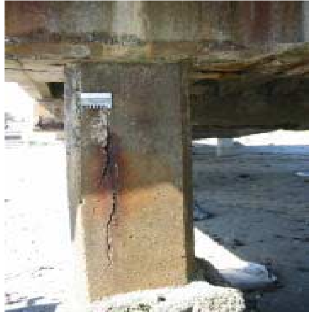
Figure 2: Vertical cracking in pile caused by corrosion of steel bar
